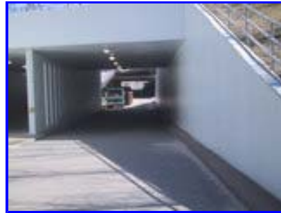
Pedestrian underpass under Nicolls Rd as see from the east (left) and west (right)
