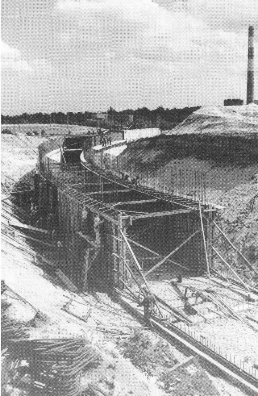
View during construction of world's largest photo synchrotron, which went into operation in 1960 at Brookhaven National Laboratory. Photograph, courtesy BNL.
