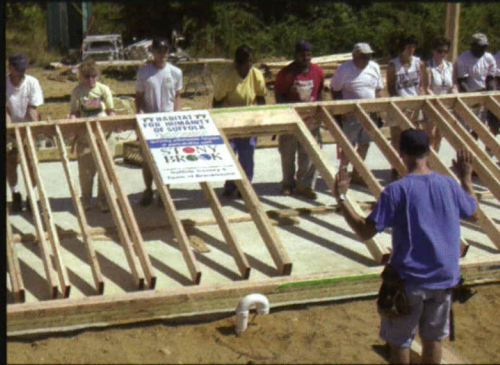
The first wall goes up, and a house starts to take shape.
