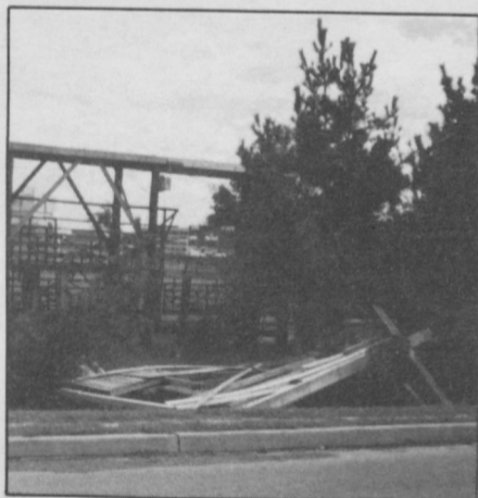
Press box demolished. The 24-foot-long press box lies in shambles near North Loop Road. Physical Plant crew members were busy rebuilding it this week for Saturday's home football game with Worcester State.
