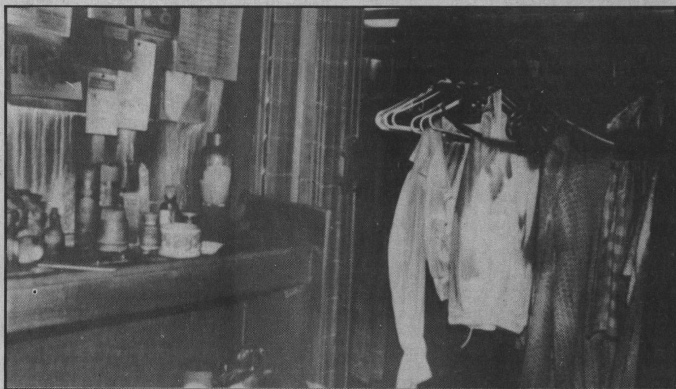
Two doors away from where the fire originated, soot and smoke residue cover clothes and personal belongings in C room of Suite 212.
