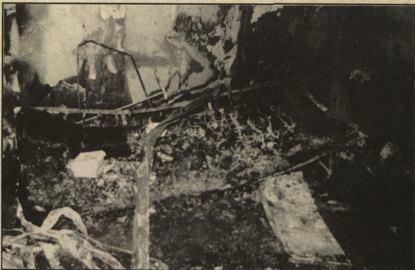
A twisted bed frame sticks out from the wreckage in suite 212A of A wing of Dreiser College, where a fire broke out last Tuesday. Arnold Gallardo/USB Weekly
