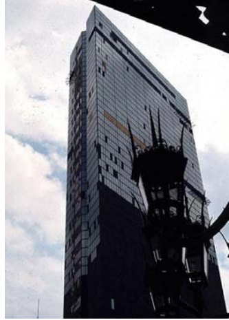
Figure 2.3 Wind induced vibration causes the fall of window glass on Hancock Tower (Schwartz, 2001).
