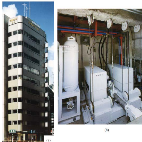
Figure 3.6 Building with active TMD. (a) Kyobashi Siewa Building (b) its active TMD unit (Kareem et al. , 1999)
